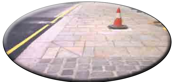
Appropriate materials should be used and cut to positively respond to obstacles
