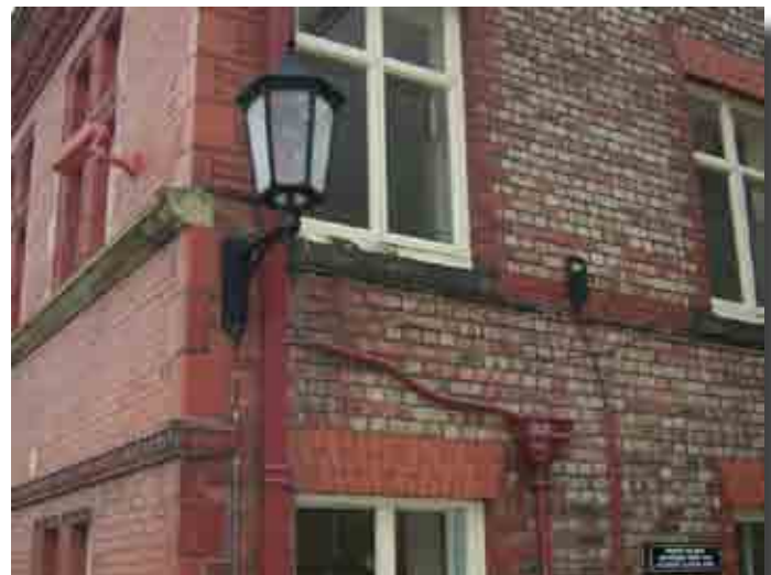
Signs, security cameras and signs will be mounted to buildings or grouped together to reduce street clutter
