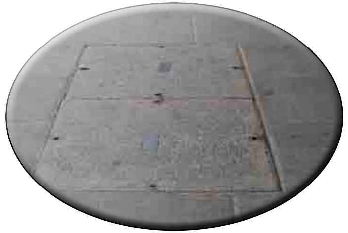
Utility grates and paving flags should not be 'plastered' with mortar
