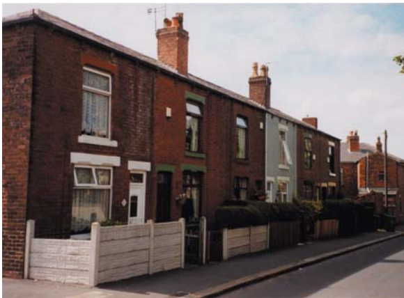
Peter Street. The replacement of timber box sash windows and doors and the removal of mullions from ground floor windows has destroyed the original unity of the terrace. The erection of concrete boundary walling and fences detracts from the streetscape
