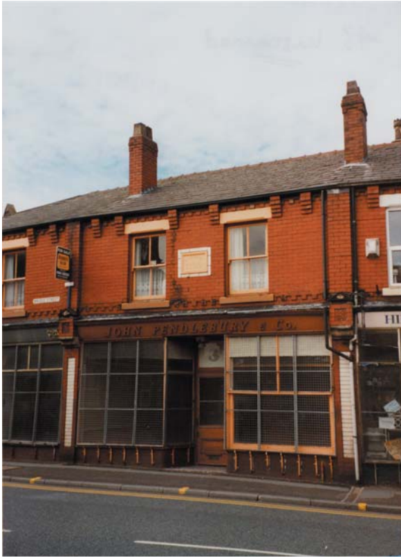
A vacant shop in Bridge Street, dated 1907 with original shop front intact, awaiting re-use.
