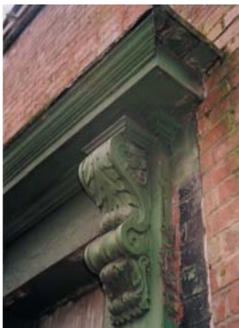
No.22 Bridge Street. A surviving late Victorian shopfront with high quality joinery
