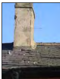
Photograph 29: Failing roof tiles
