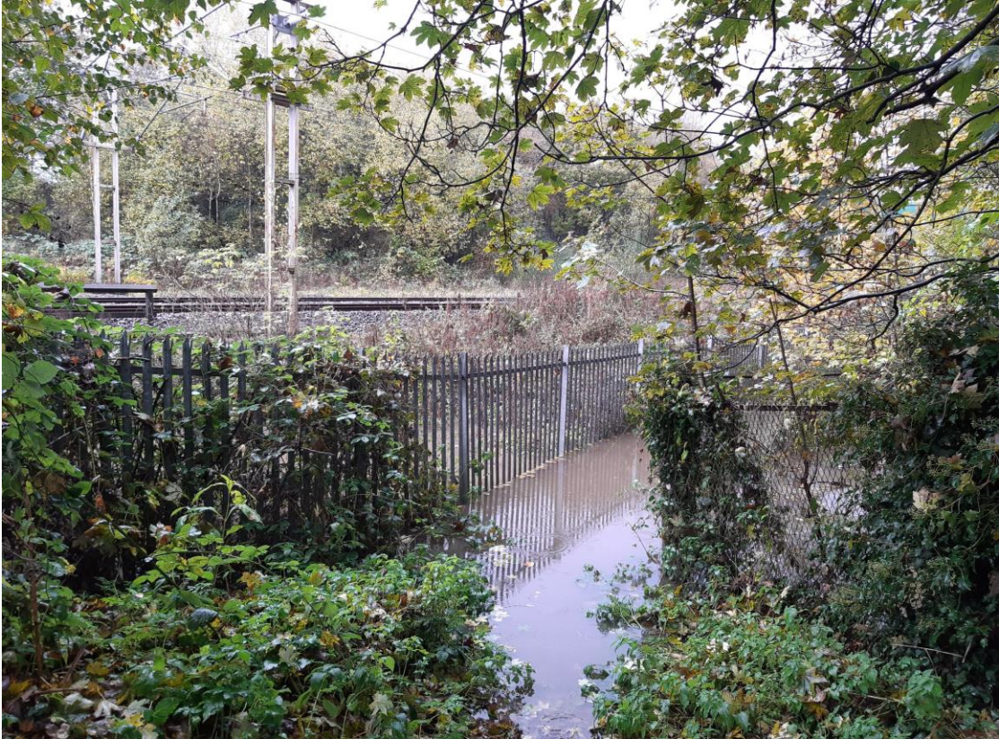
Figure 2 - Flooding at Inlet to Network Rail Culvert (Morning 06/11/2023) Facing Downstream.
