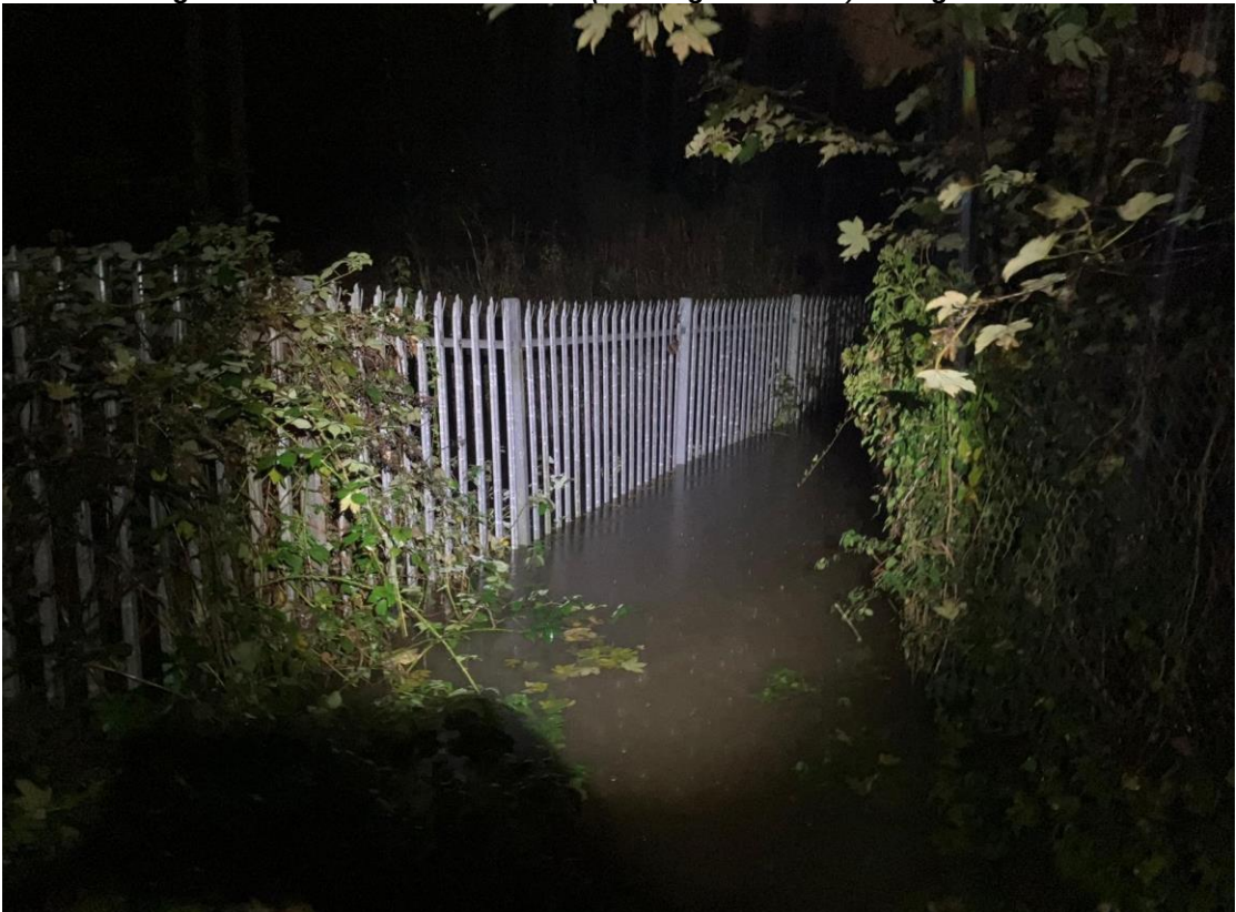
Figure 3 - Flooding at Inlet to Network Rail Culvert (Evening 06/11/2023) Facing Downstream.
