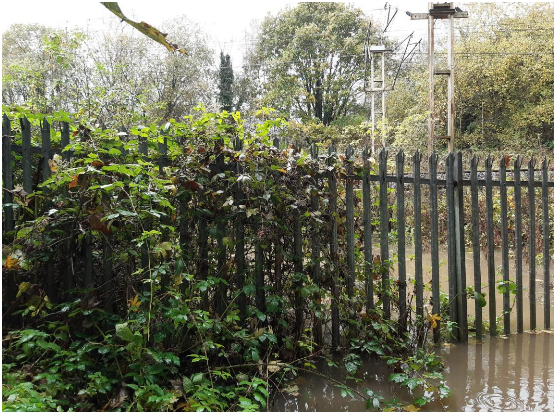
Figure 1 - Flooding at Inlet to Network Rail Culvert. Inlet is submerged. Facing Downstream
