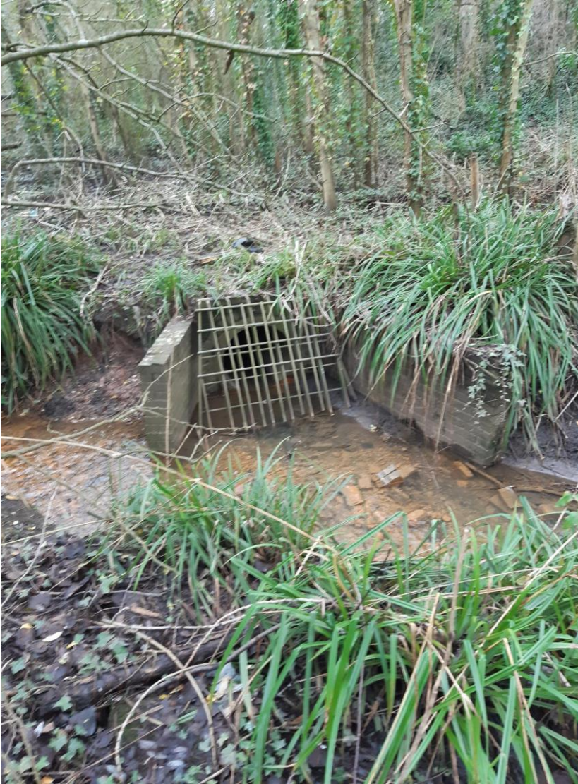
Figure 7 - Outlet of UU Surface Water Sewer Under Normal Conditions. Upstream of Network Rail culvert. Winter 2024.
