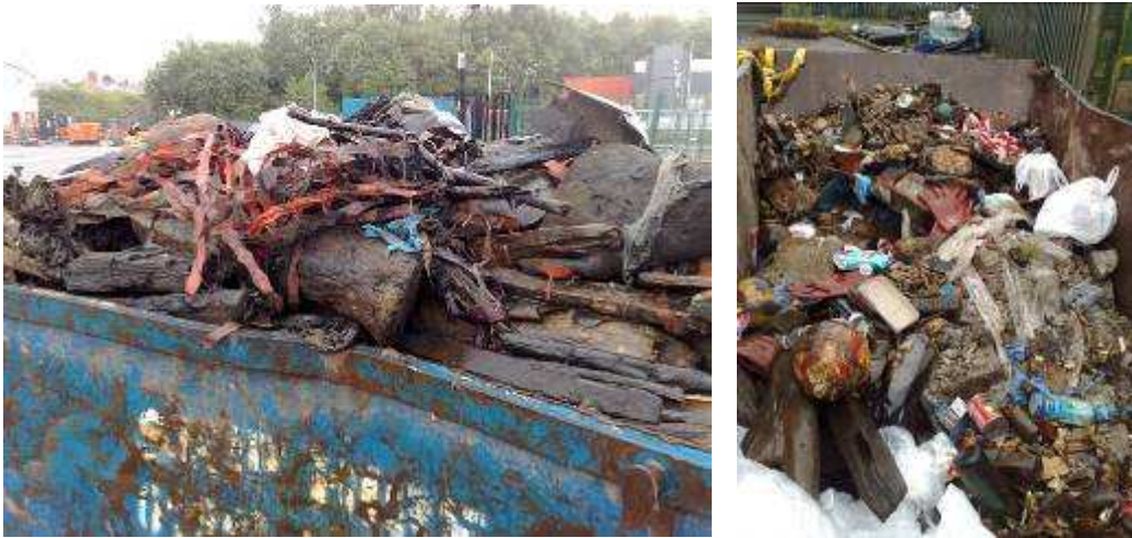
Figure 4 – Debris removed from Culvert
