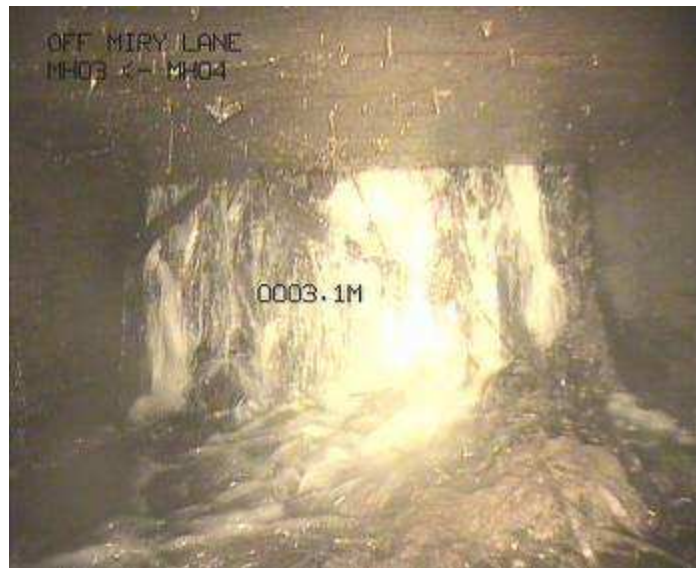
Figure 3 – CCTV Screen shot of Blockage
