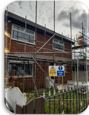
Picture: Repair works to a property purchased as part of the Golborne and Lowton purchase and repair scheme
