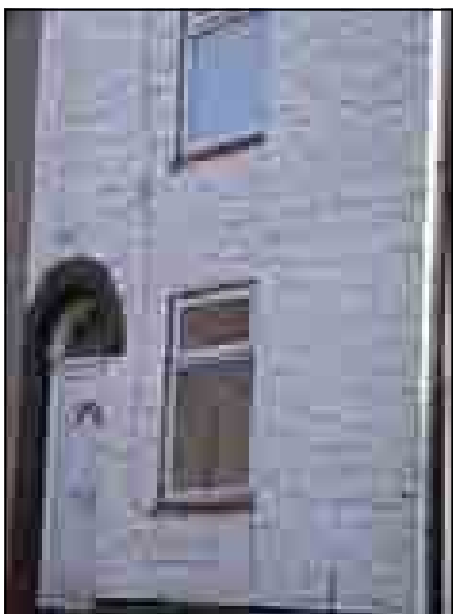
Photograph 8 (above): Example of concrete render found on several properties within conservation area.
