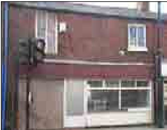
Photograph 38: 170 Elliott Street, old laundrettes. Has lain empty for some time and suffering from lack of use.
