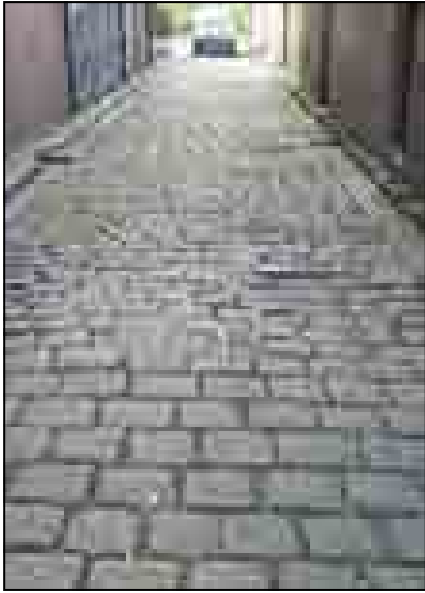
Photograph 35: Example of intact sets along back alley. Positive enhancement of the streetscape.
