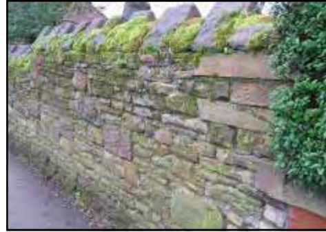
Photograph 32(right): Traditional stone built wall which survives in the centre of the conservation area
