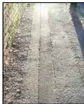
Photograph 27 (above): More poorly maintained paving surfaces within conservation area.
