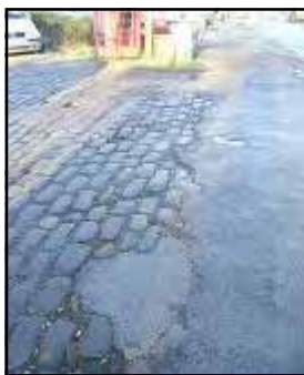
Photograph 25 (above): Poor quality street surfacing at entrance into Balcarres Arms car park.
