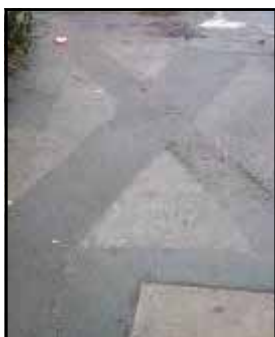
Photograph 26 (below): Poorly repaired paving surface within conservation area.
