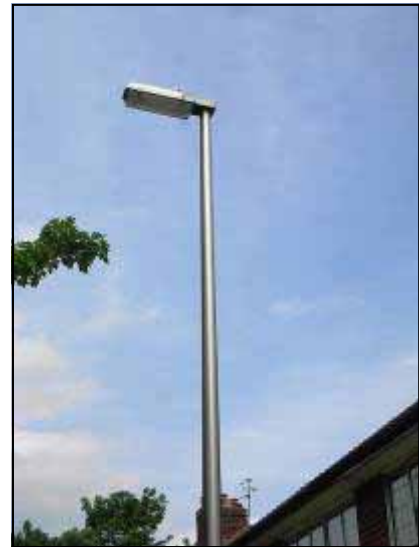
Photograph 20 (right): Lighting column along St Helens Road.
