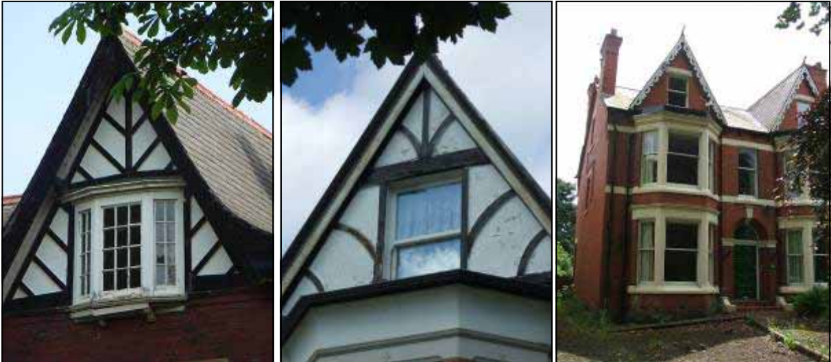
Photographs 27 & 28 (left & centre): Examples of maintenance issues within conservation area. Both photos show peeling paintwork and rotting wood.
