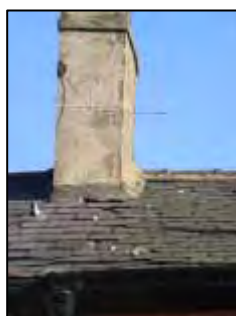
Photograph 29: Failing roof tiles
