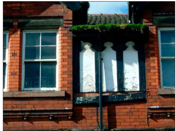
Poor maintenance on Gerard Street.
