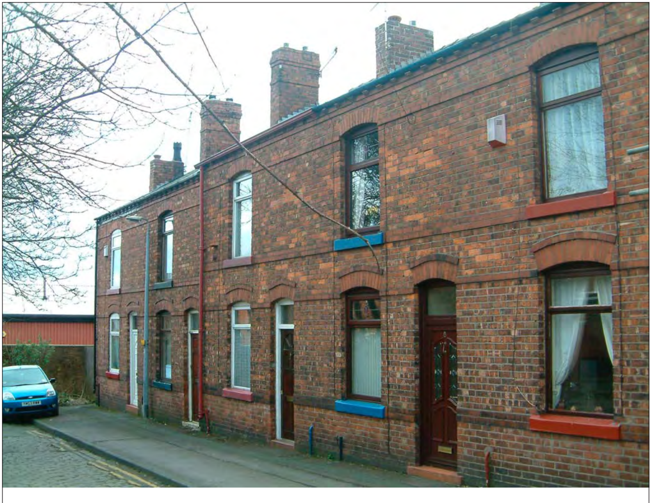
A Court terrace with replacement doors and windows detracting from the original brick detailing.
