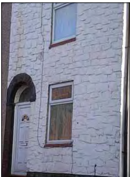
Photograph 8 (above): Example of concrete render found on several properties within conservation area.
