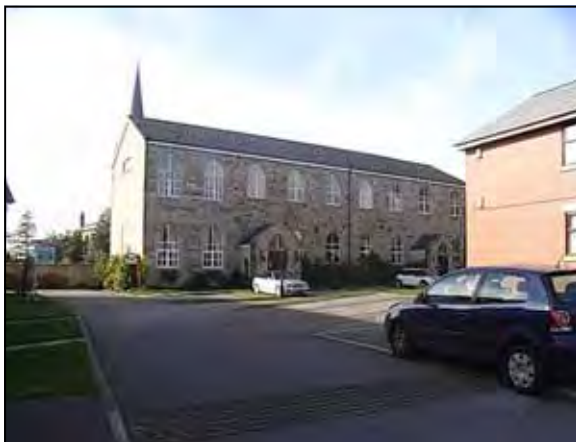
Photograph 41: Conversion of Tyldesley Church School to apartments with new building in foreground.
