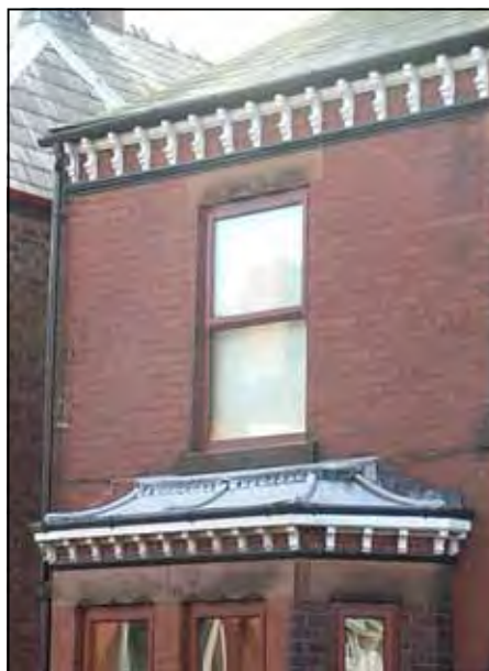
Photograph 9 (below): Example of corbelling detail. This is quite a very ornate example.
